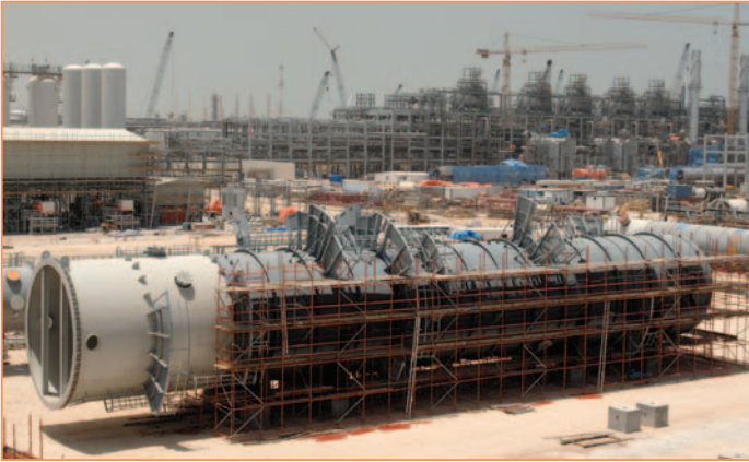
Sulfur recovery area
