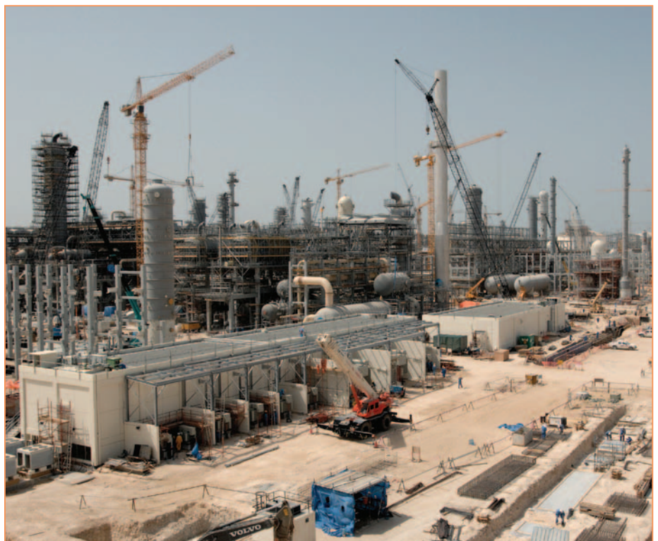
Train 5 Sulfur recovery units
